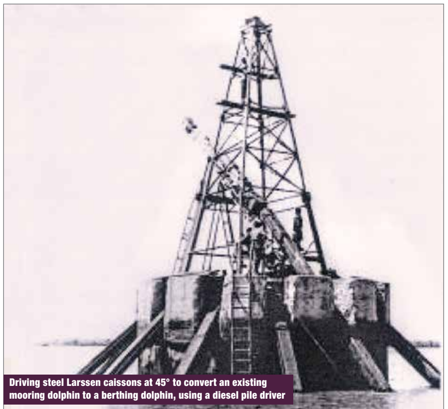
Jack-up floating platform carrying 50 tons of piling equipment, used in the construction of the Matola dolphins
