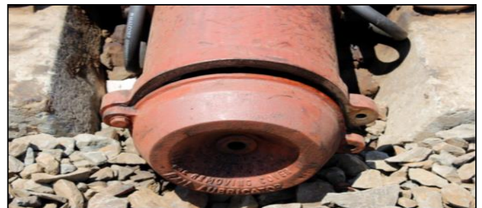
Figure 6. Incorrect Maintenance Practice for Grease Refill
