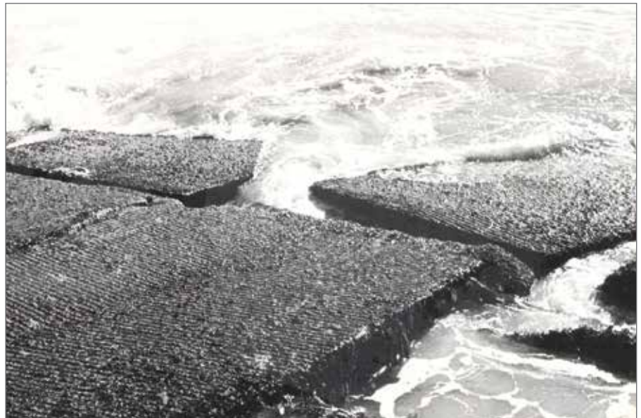
Photo 7: Break-up of Yzerfontein ramp, 1978
