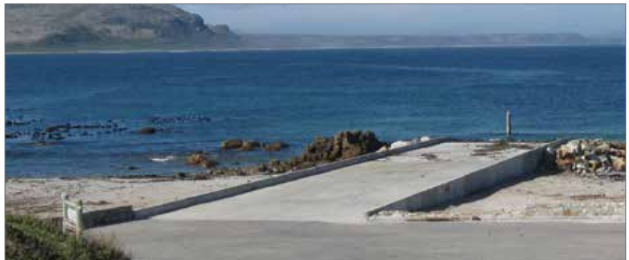
Photo 6: Witsands ramp 2008 – long approach to get correct end grade and end depth
