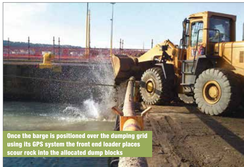
A front-end loader busy stockpiling rock on the jumbo barge in preparation of the journey to the desired berth
