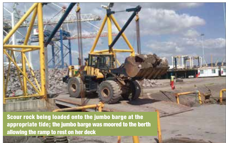
Specially designed ramp used to load material from the stockpile onto the jumbo barge at Berth 205
