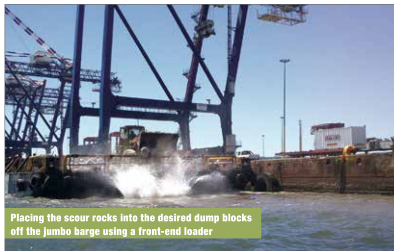
The jumbo barge is held in position over the dumping grid using her mooring and winch systems during the dumping operation
