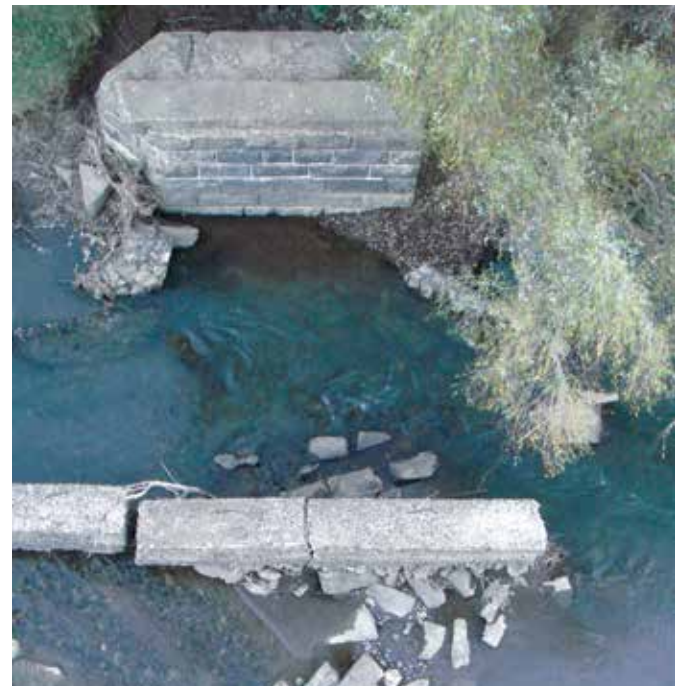
Figure 10: Some of the old pier foundation remnants of the first 1905 permanent bridge (#2) are still visible directly below the 1926 permanent bridge (#7) (Photo Bertus Bekker 2014)
