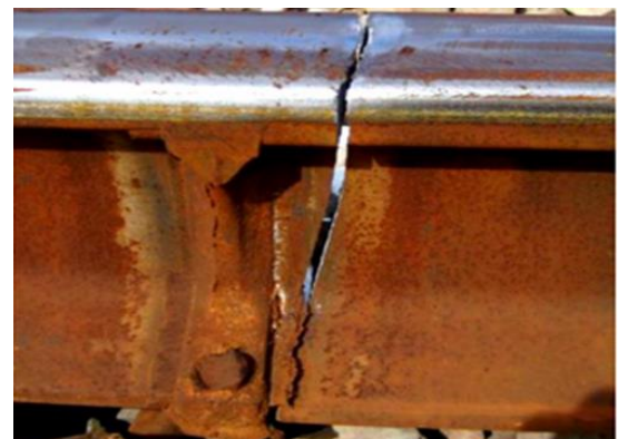
Figure 1: Transverse failure adjacent to the weld
